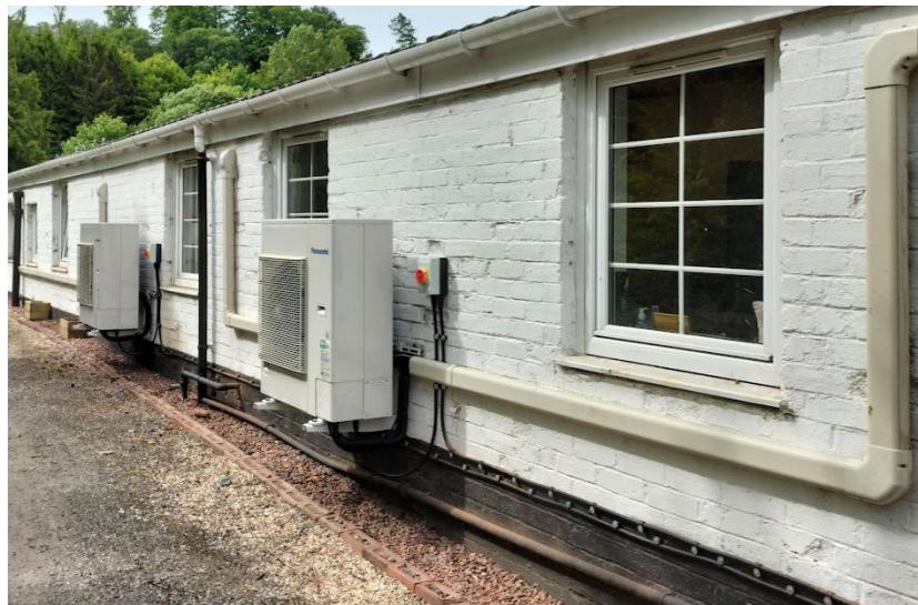
Air to Air units on community building used intermittently
