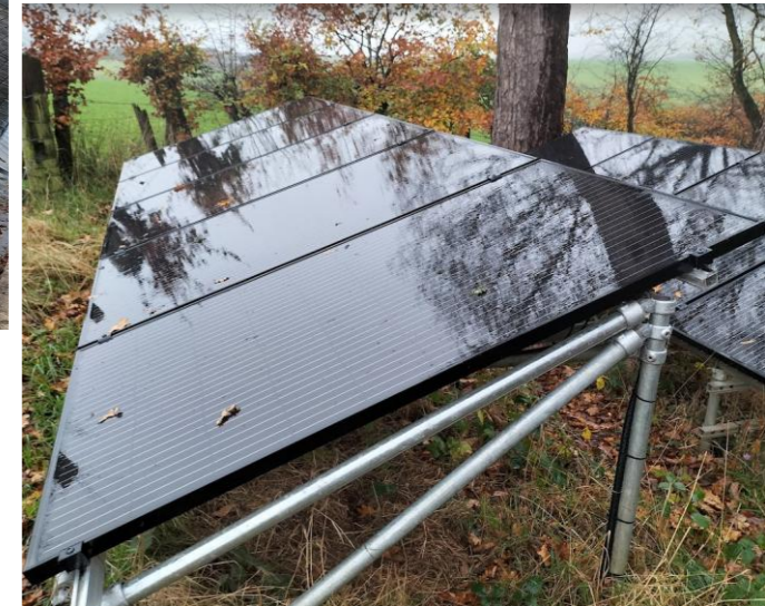
Roof mounted PV in a conservation zone on rear facing roofs on left and ground mounted array away from the building on the right
